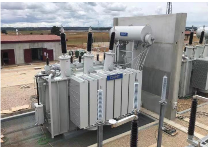
Greece | Terna Wind Farm 150kV Power Transformer Project
