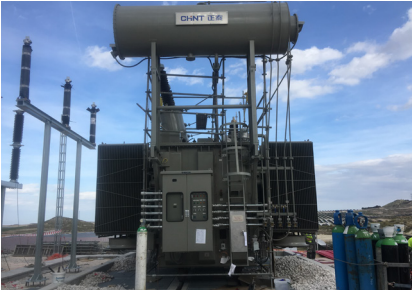
Spain | Maetel 5.6MW Solar Power Plant
