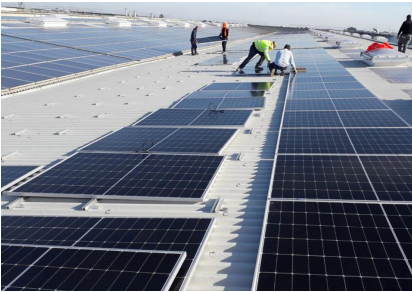
Italy | CARTON PACK S.p.a. 2MW Rooftop Solar Plant
