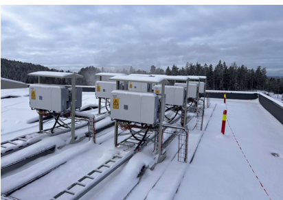
Norway | 2MW Rooftop Project
