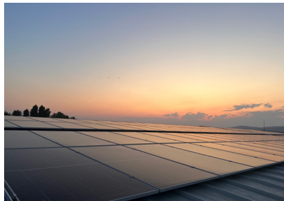
Azerbaijan | Winery 450kW Rooftop Project
