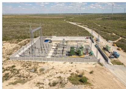
Mexico | Reynosa wind power station 400kV 225MVA Power Transformer Project
