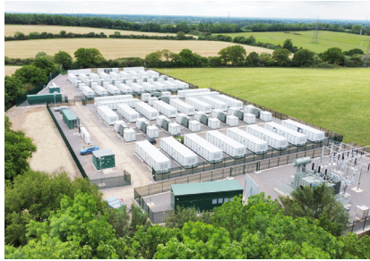
UK | Minety 99.8MW/98MWh BESS Project
