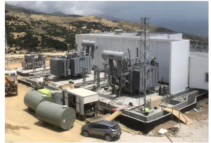
Greece | METON New Energy Power Station Transformer project
